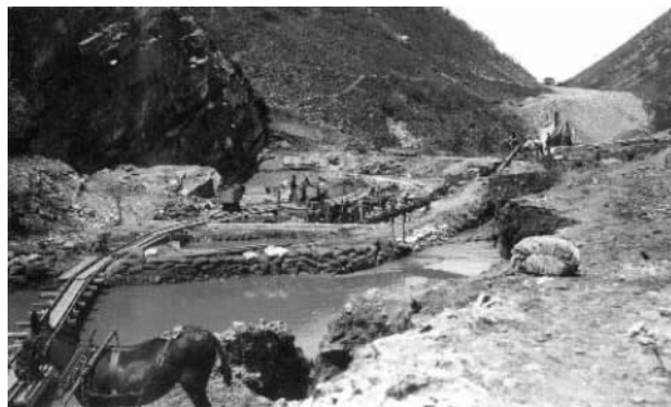
Photograph 2. Reclamation Service pushed the construction of the power system (including the Spanish Fork Diversion) to provide electricity for tunnel construction. Circa 1907.
