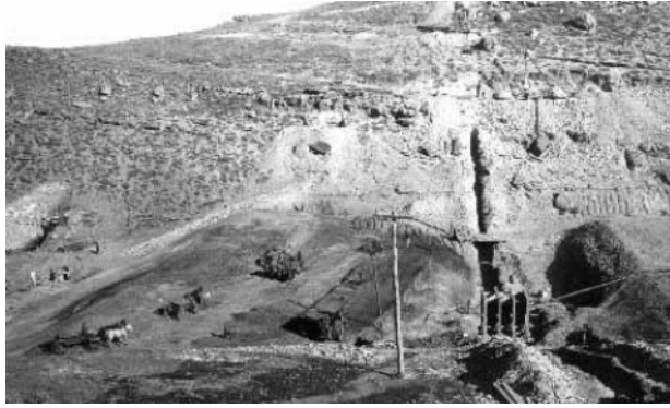
Photograph 7. While horse-drawn wagons delivered thousands of loads of earth fill to the Strawberry Damsite, the core wall trench was being excavated. Circa 1911.
