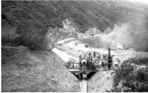
Photograph 3. The majority of the Power Canal traversed steep slopes and had to be concrete lined. Circa 1907.
